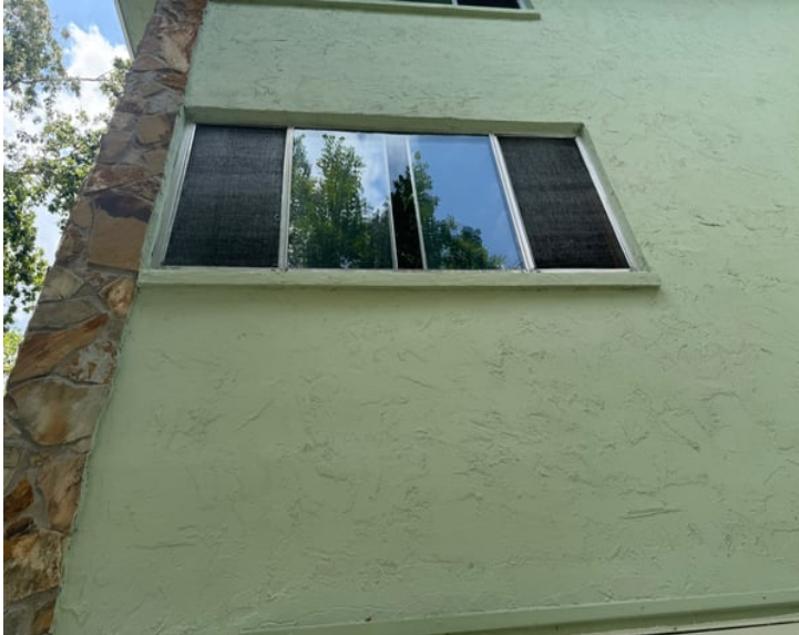
Stories 1-3 - Common Areas: Glazed (Protection Level-X)
