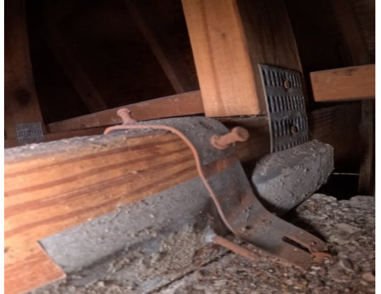
#2 toe nail- gap greater than 1/2"
