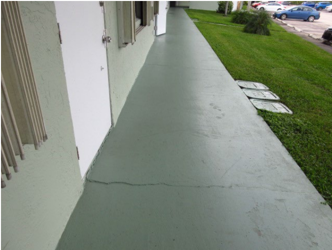
VIEW OF CRACKS AT GROUND LEVEL WALKWAY
