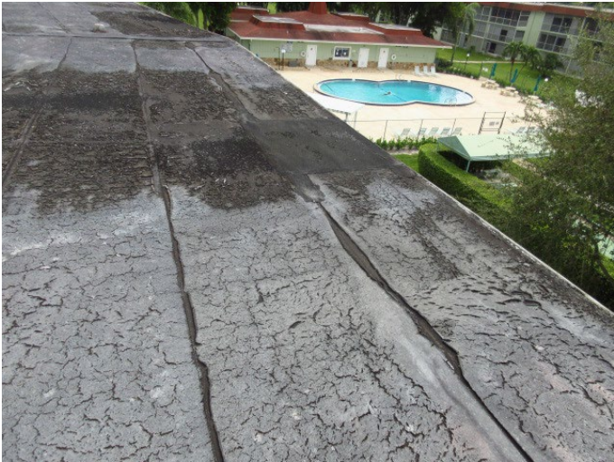
VIEW OF FAILING ROOF MEMBRANB
