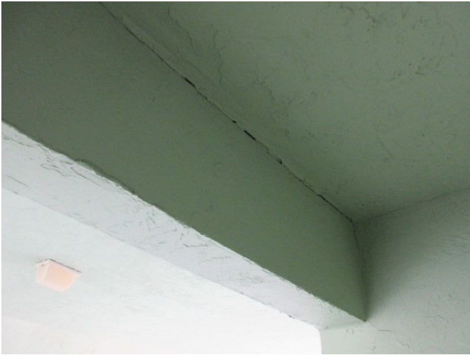
VIEW OF CRACKS AT SLAB UNDERSIDE
