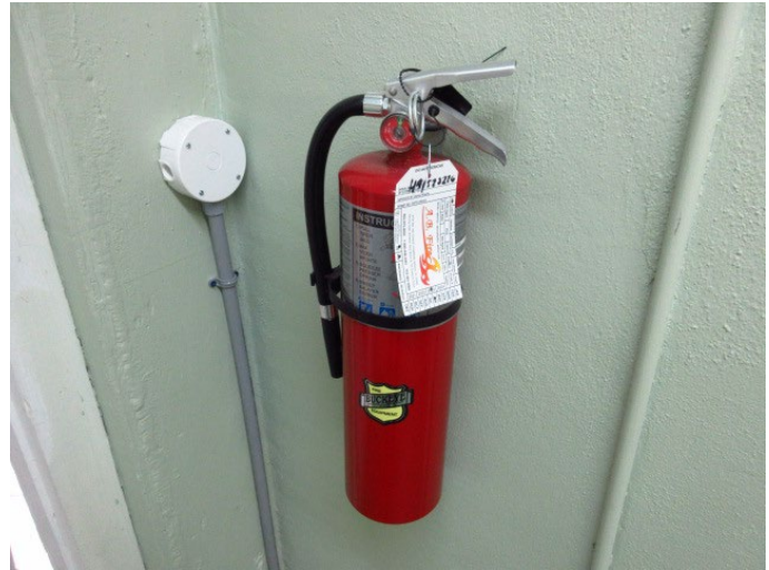
VIEW OF FIRE EXTINGUISHER
