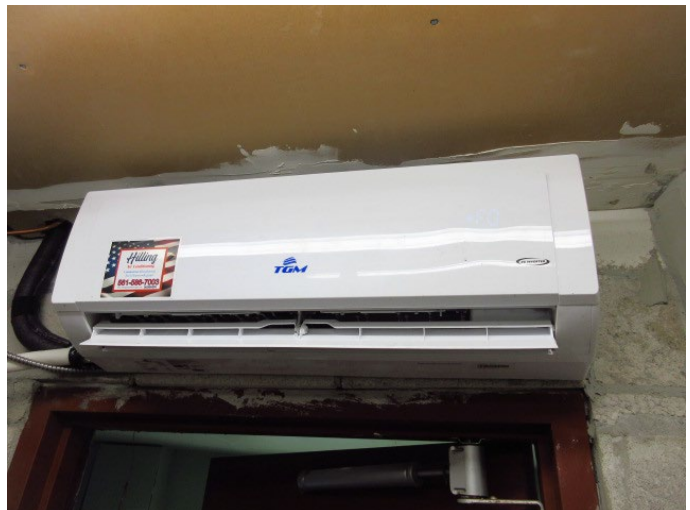
VIEW OF ELEVATOR ROOM A/C UNIT
