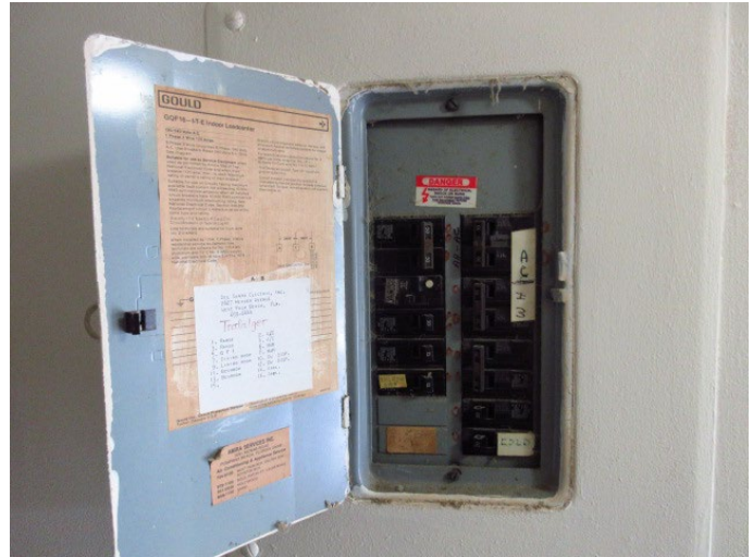
VIEW OF ELECTRICAL EQUIPMENT
