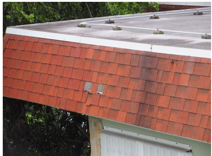
VIEW OF DAMAGED / . MISSING MANSARD SHINGLES
