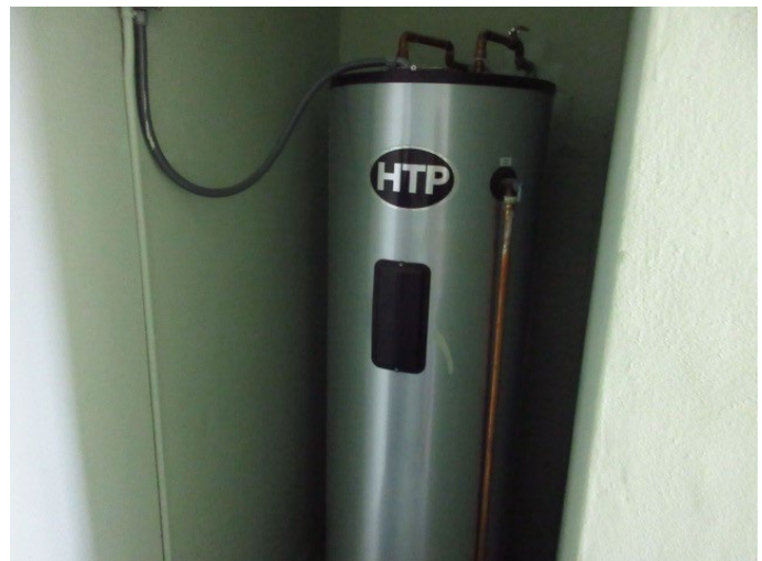
VIEW OF COMMON AREA WATER HEATER
