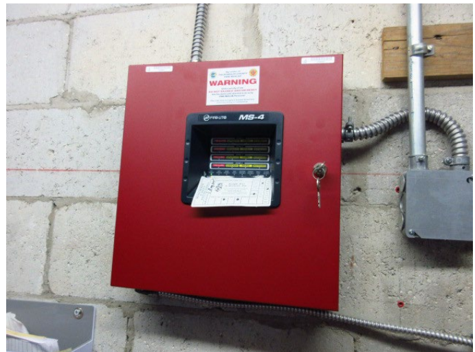
VIEW OF CENTRAL ALARM PANEL
