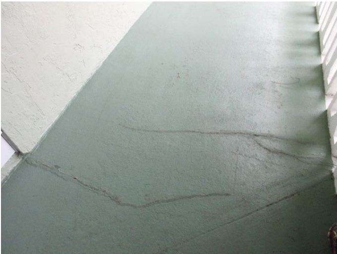
VIEW OF CRACKS AT ELEVATED WALKWAY
