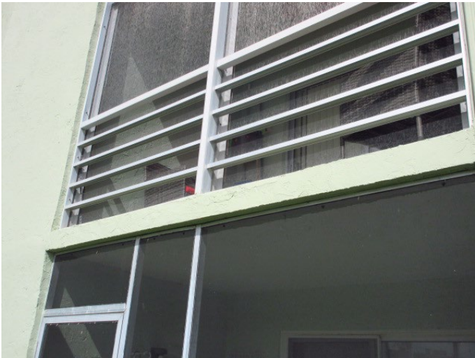
VIEW OF CRACKS AT BALCONY DECKING
